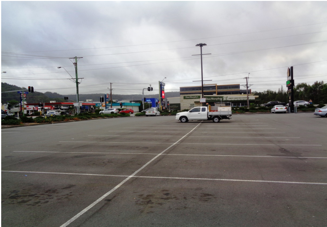
Photo 1 - Site, looking toward the north, minor oil staining on asphalt pavement, 29 Jan 2018.
